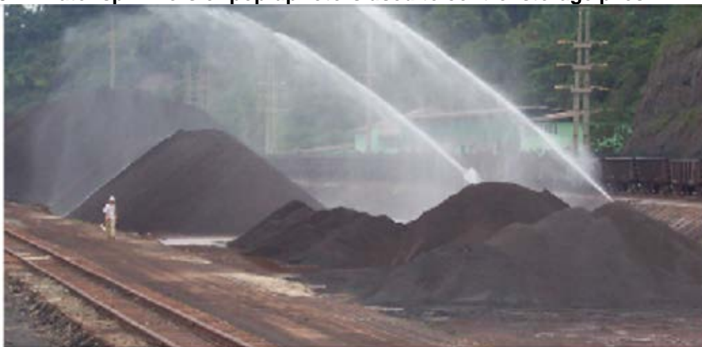
Figure 5-1: Water sprinklers or pop-up rotors used to control storage piles
