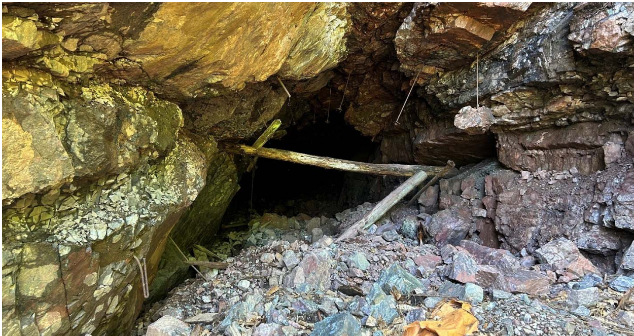
Photograph 1 – Adit proposed for rehabilitation. Note the presence of fallen timber and rocks indicating failure of the adit brow and crown pillar (June 28, 2023).
