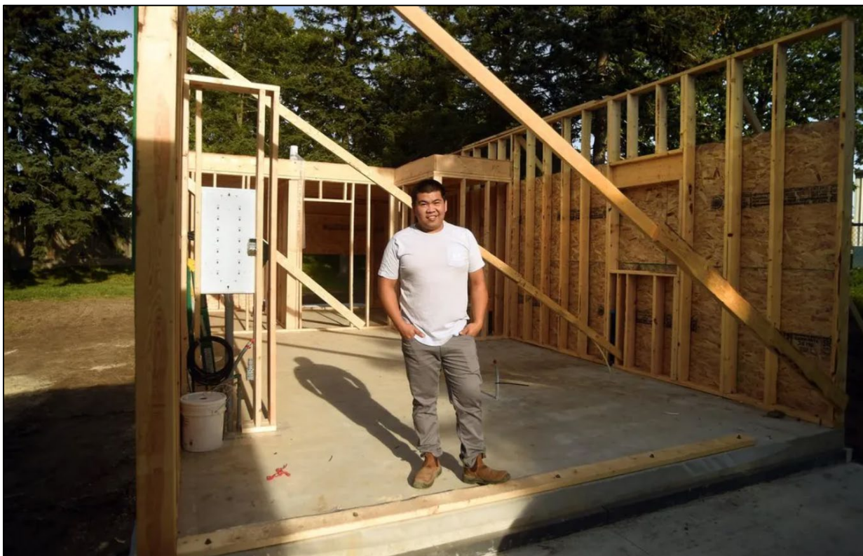
2021 tiny house under construction in Kitchener (photo source: David Bebee / Waterloo Region Record )
